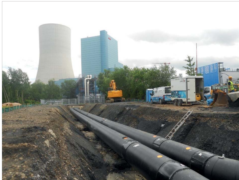
Figure 2. Start of pipe route after service pipe bridge at newly constructed power plant with mounted casing joints
