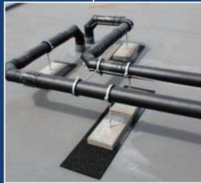
The many daily movements are absorbed in the bends, designed for this purpose, just like the pipe supports absorb forces.
